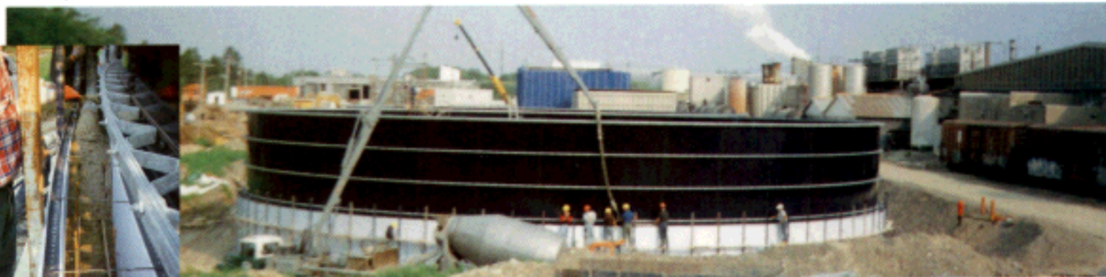
McCain Foods: Potato Waste Water Treatment Tanks - "We installed two treatment tanks for McCain Foods that were 112 ft. in diameter and embedded 10 ft. below grade. We chose ICFs for the project. As well as an insulating advantage, the ICFs offered excellent protection for our glass lined tanks. The building process was very versatile and quick to install." Nelson Ward, Greatario Industrial Storage Systems
